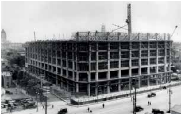
The Hudson Bay Company building in Winnipeg, on which Alexander Scott, 1.3.3.3a, worked, under construction, 4 June 1926
